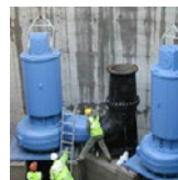
IRELAND Maintaining pressure at pumping stations
